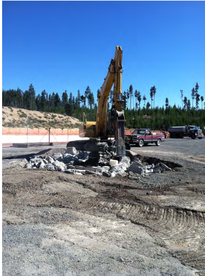
Figure 2-13. Excavation of NWG 55-29 cellar in preparation for the modification of the wellhead for new 30.48 cm (12 in) Series 1500 valve. The valve pictured is the original Series 900 valve installed by Davenport Newberry after well drilling.
