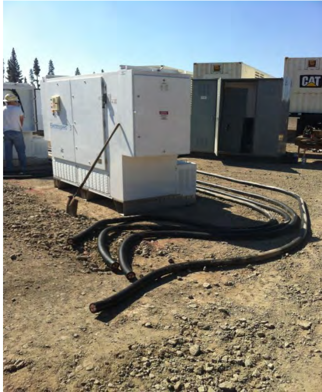
Figure 2-27. Installation of VSD 1 (white box in foreground). The gray box behind VSD 1 is a dedicated breaker cubicle for the VSD. The armored cabling that connected 460V phases between the cubicles and then the 800HP pump drive is placed on the ground prior to termination.
