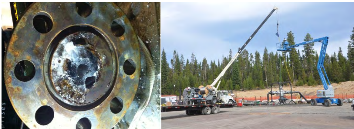
Figure 3-8. Left: ice in the lubricator after removal. Right: the lubricator on top of the wellhead (thin green object) and boom crane with basket.
