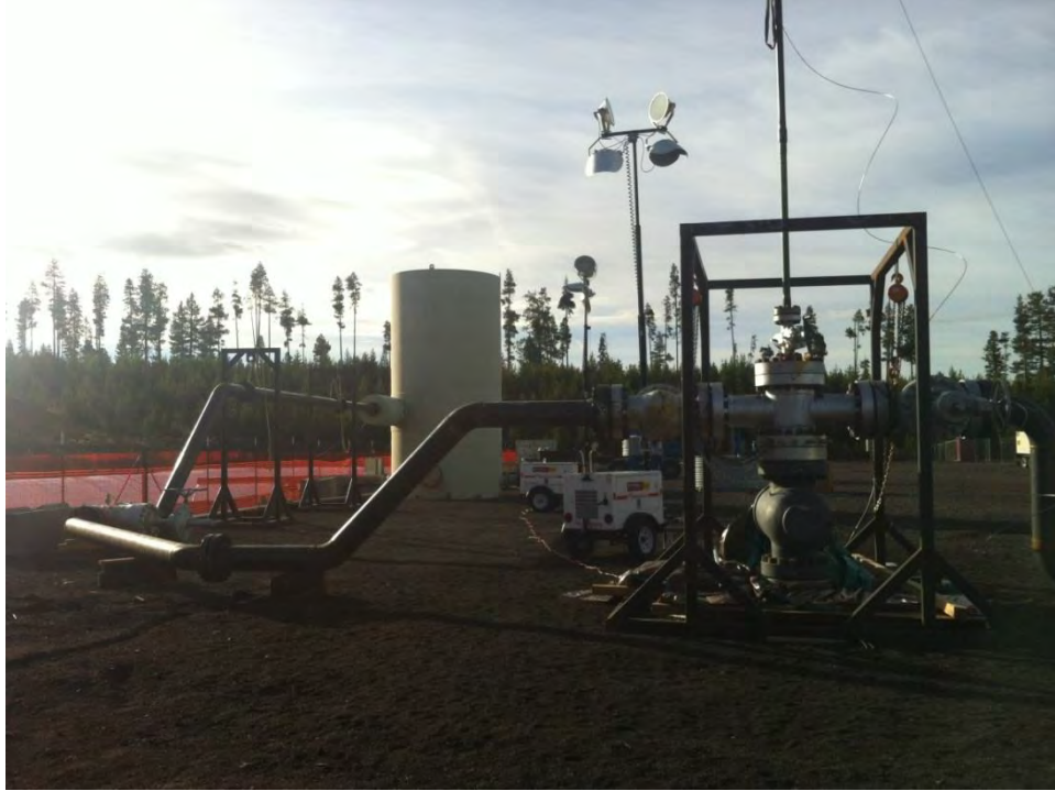
Figure 2-30. Flow back piping, phase separator (large white cylinder) and wellhead.
