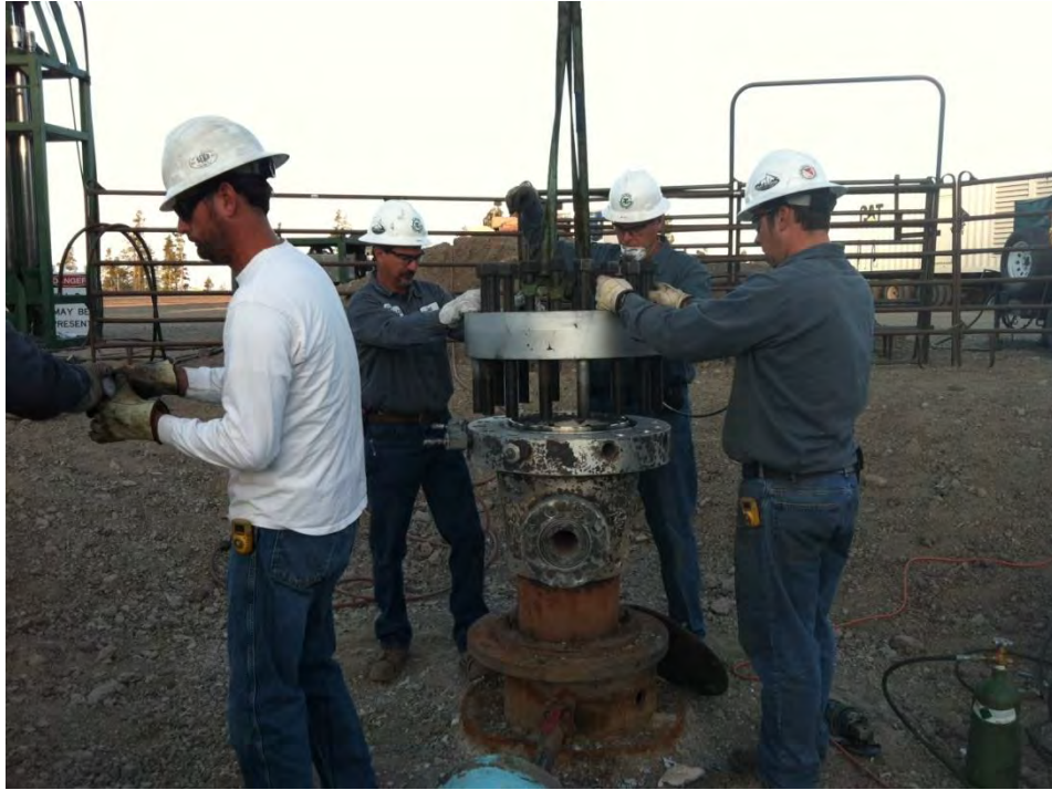
Figure 2-14. The new wellhead adapter being installed on existing 34 cm (13 3/8 in) casing; the mottled surface of the adapter was due to in-place weld heat-treatment. TNG personnel are installing the 30.5 cm (12 in) double studded adapter prior to the installation of the new 30.5 cm (12 in) Series 1500 Wellhead valve.
