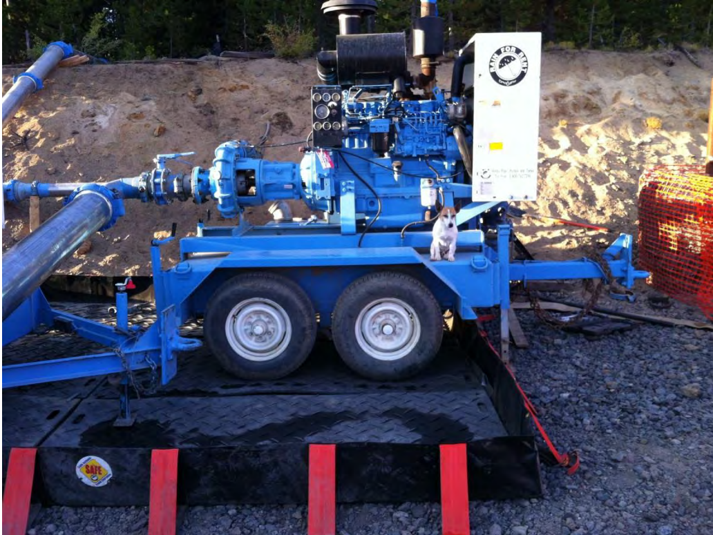
Figure 2-24. Model 3HA high pressure pumps used to pump water uphill to Pad S-16.
