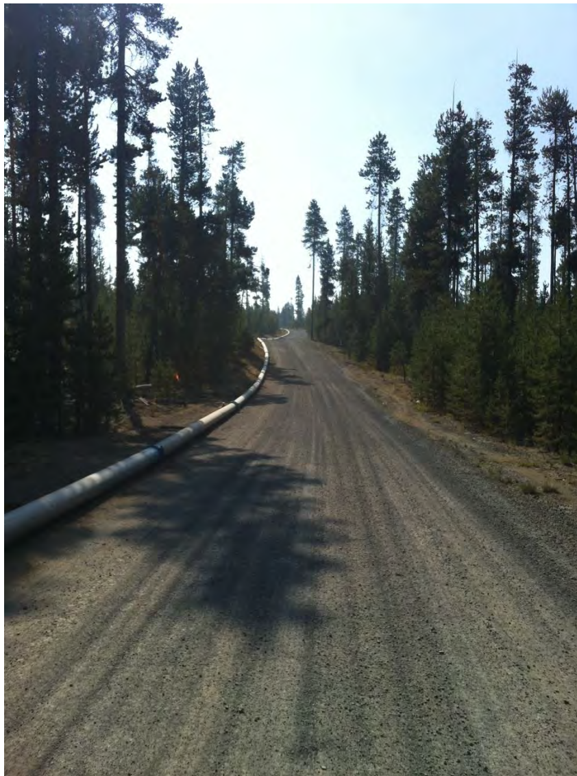
Figure 2-23. Roadside construction of the backup water supply pipeline from Pad S-16 to Pad S-29.
