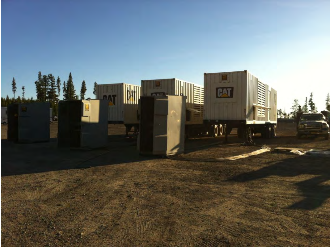
Figure 2-26. Initial set up of XQ1000 generators (large white containers). From left to right they are labeled Generators 1, 2 and 3.
