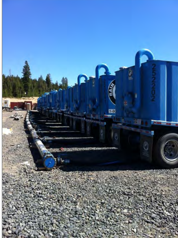
Figure 2-21. Water storage tanks connected to 25 cm (10 in) header line.
